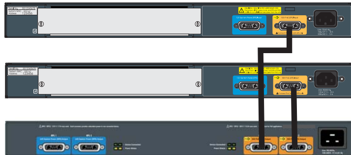
Figure 2-14. Connecting EPS to 2, 24 port switches.
